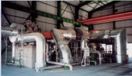
Air compressor and gas expander for P.T.A. plant
