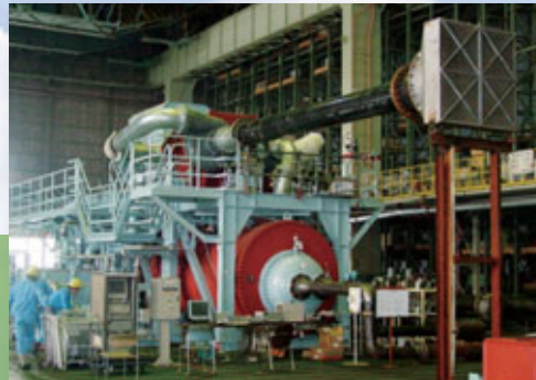
Booster air compressor for Power Station IGCC
