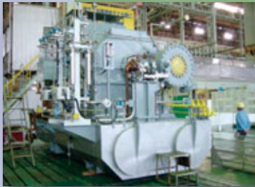
Fuel gas compressor for Power plant
