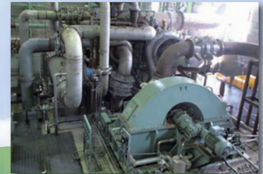
Air compressor and gas expander (Combined type) for P.T.A. plant
