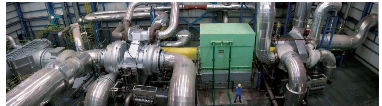
Air compressor (6-stage) and gas expander for PTA plant
