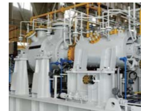
Gas Injection Compressor for FPSO
